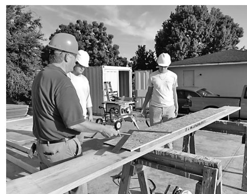
Ten seniors with The Villages High School's Construction Management Academy will help Habitat for Humanity build a home this school year. Submitted photo
